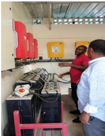
WeTu Solar Battery Storage unit
